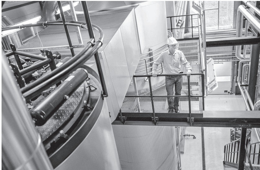
Jens Dall Bentzen at a furnace in Sonderborg, Denmark, that is built on a design he developed with a government grant. It burns organic matter to generate heat.
