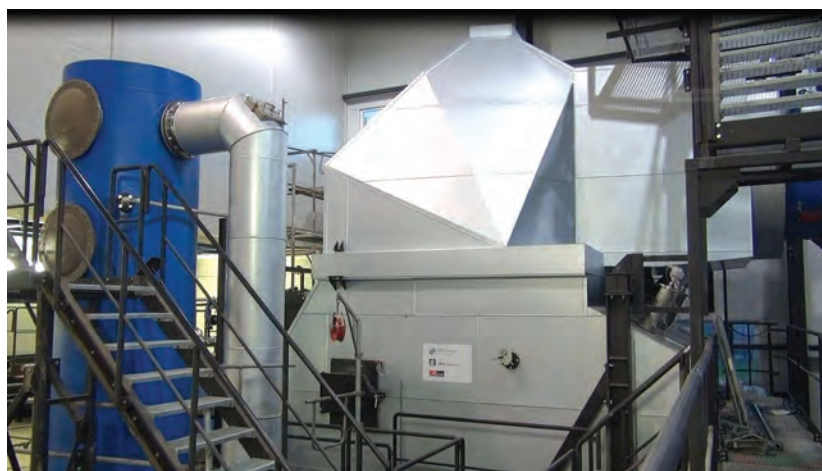
The 8 MW demonstration furnace at Bogense Fjernvarme heating plant
