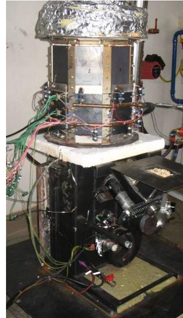
Pellet boiler with TEG 250 fuel input 10 kW th , 170 W el [103]
