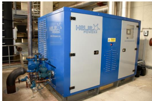
Figure 24: Heliex GenSet installation in Obertrum am See (A) (by courtesy of Heliex Power Ltd)
