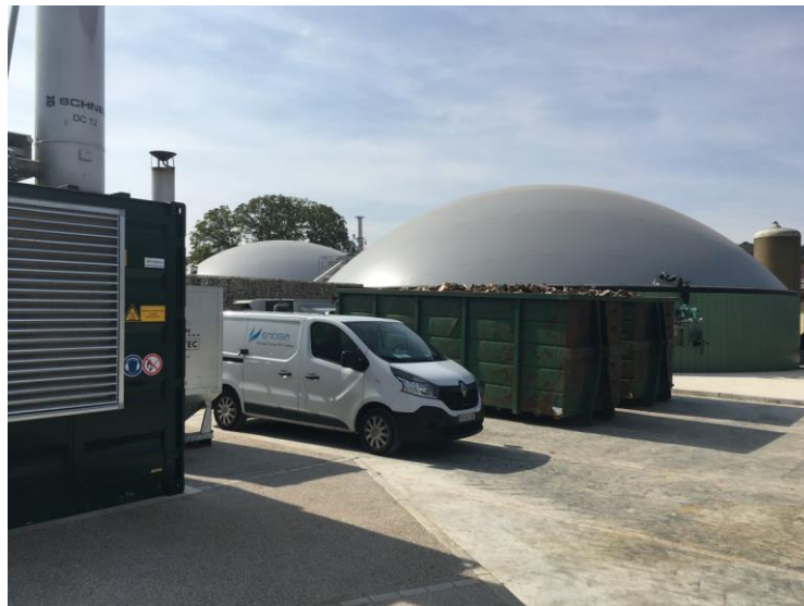
Figure 34: Biogas and wood drying installation (La foulrière, France)
