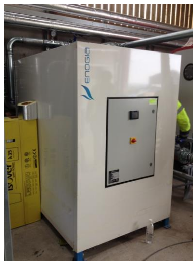
Figure 33: 40 kW machine, installed after a wood boiler
